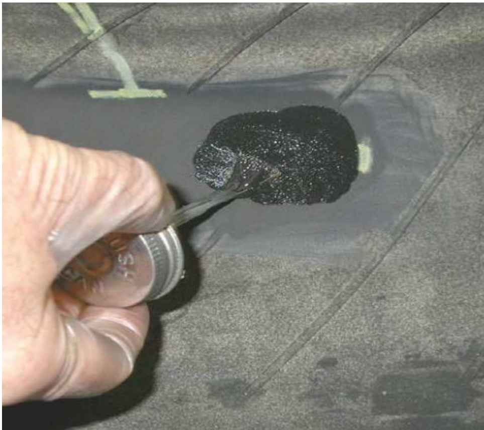
Brushing the cement both into the cleaned area and the surface of the gray gum on the patch.
